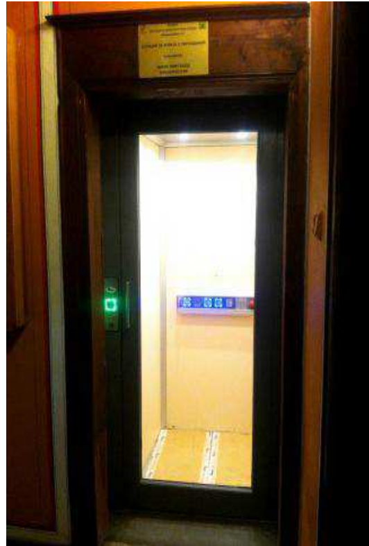
In process of installation
